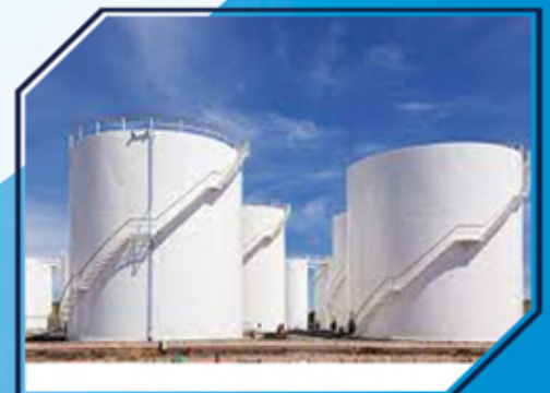
Chemical Storage Tank
