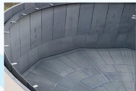
RUBBER LINING INSIDE STORAGE TANK
